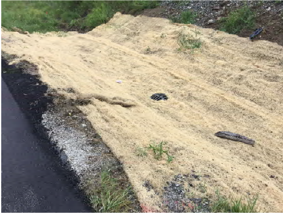
PHOTO 9 Condition Description Median drain grate between US 231 & RR
