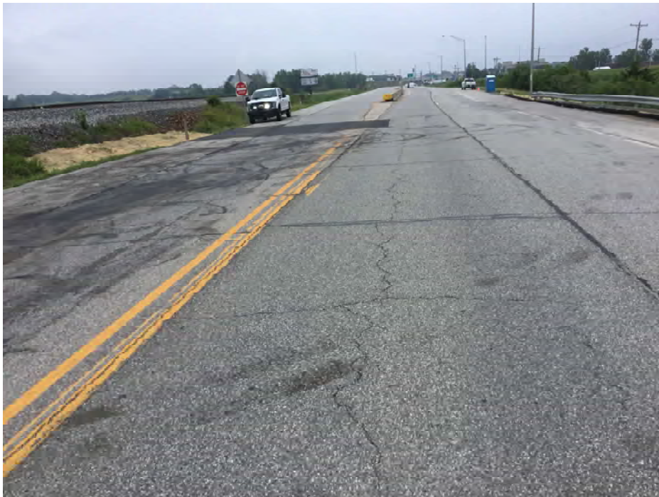
PHOTO 2 Condition Description Road alignment looking South & pavement condition above culvert
