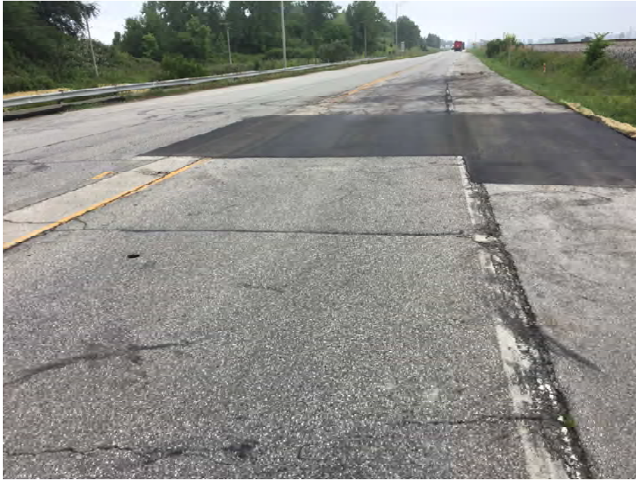
PHOTO 1 Condition Description Road alignment looking North & pavement condition above culvert
