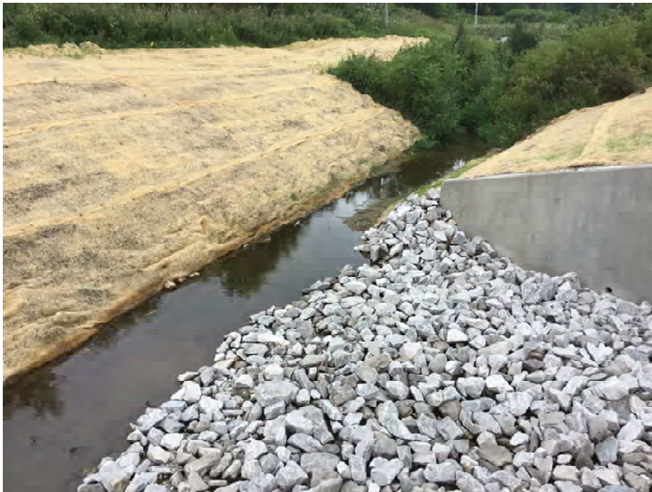
PHOTO 8 Condition Description Downstream channel flows parallel with 231 on West side of road
