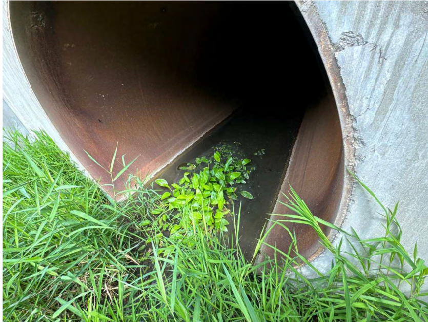
Photo 49. Taken west of US 231 facing northeast showing water entering Wetland D.
