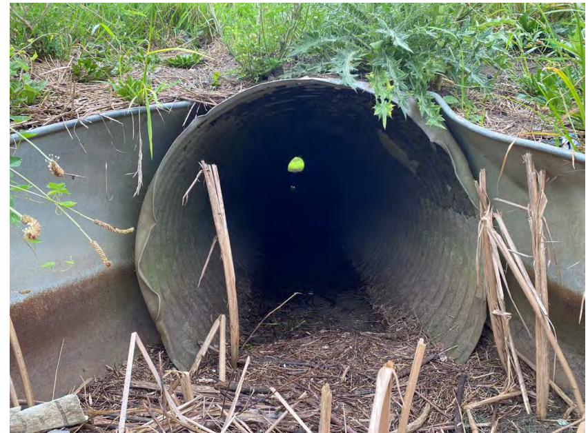
Photo 4. Taken east of US 231 facing south showing the pipe (outlet) underneath the subject drive.
